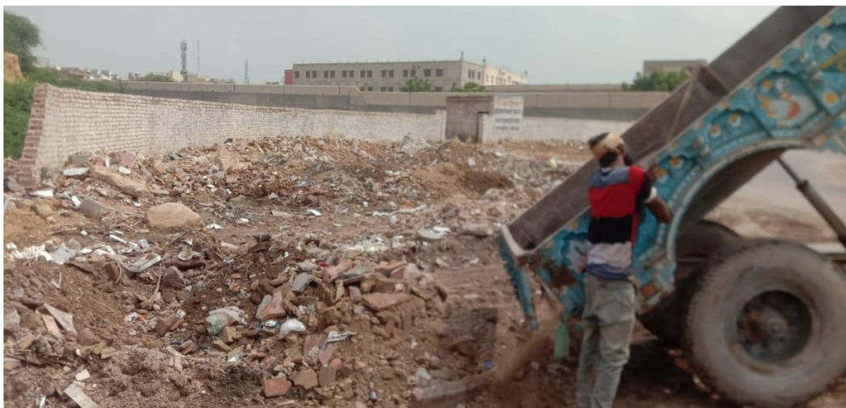
Fig. 5.2A: C&D Waste Dumping Site located in Bikaner Municipal Board (28.001359°N, 73.305546°E)
