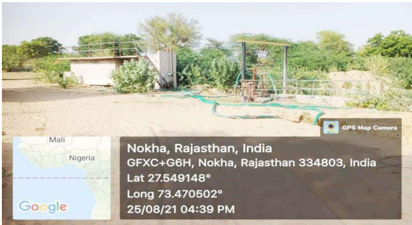
Figure 10.3: Existing STP located in Municipal Board Nokha, Bikaner (Capacity of plant is 1.0 MLD)
