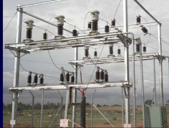
33KV Feeder to Grid
