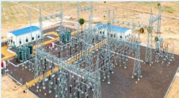
33/220 kV Hybrid Pooling Substation
