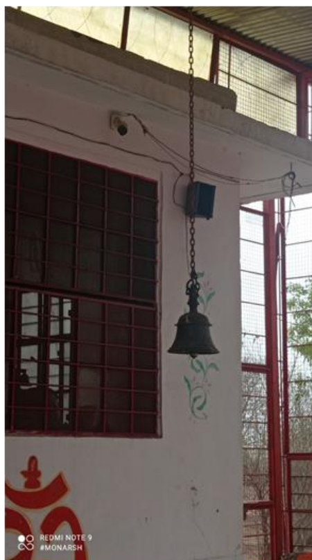
CCTV and Sound System
