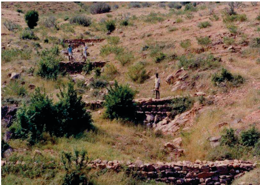
Figure 26: LSCD constructed in series in a drain
