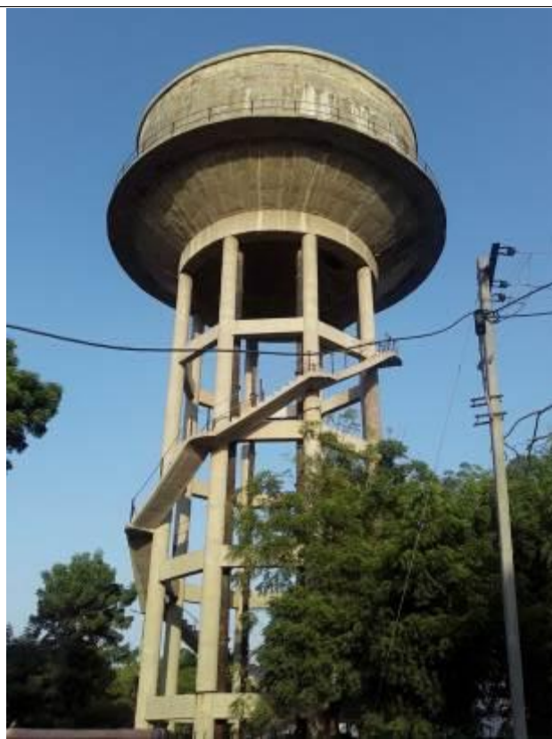
OHSR at Luni Pump House
