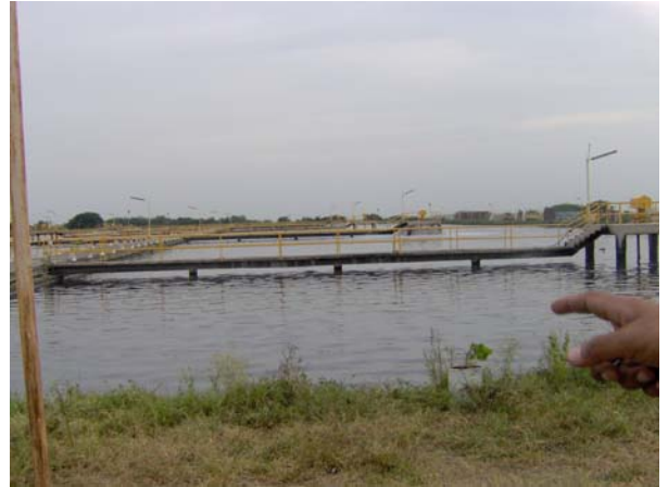
Photo 5: Typical STP Pond
