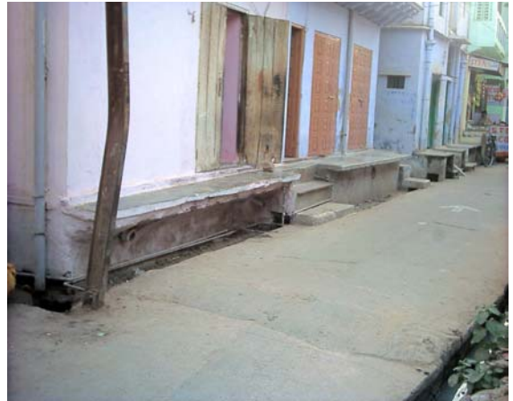
Photo 20: Encroachments into ROW
