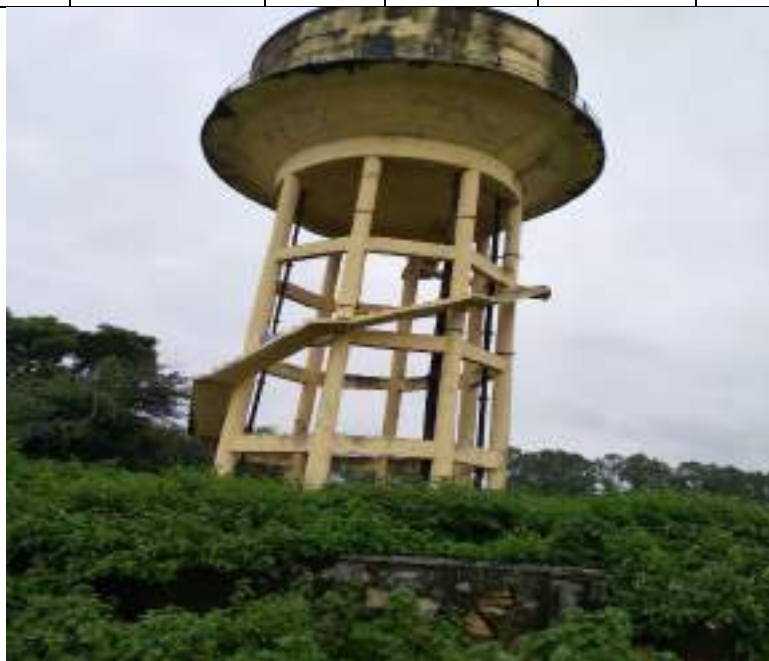
Figure 11 : Existing ESR at Navadera (325 KL)
