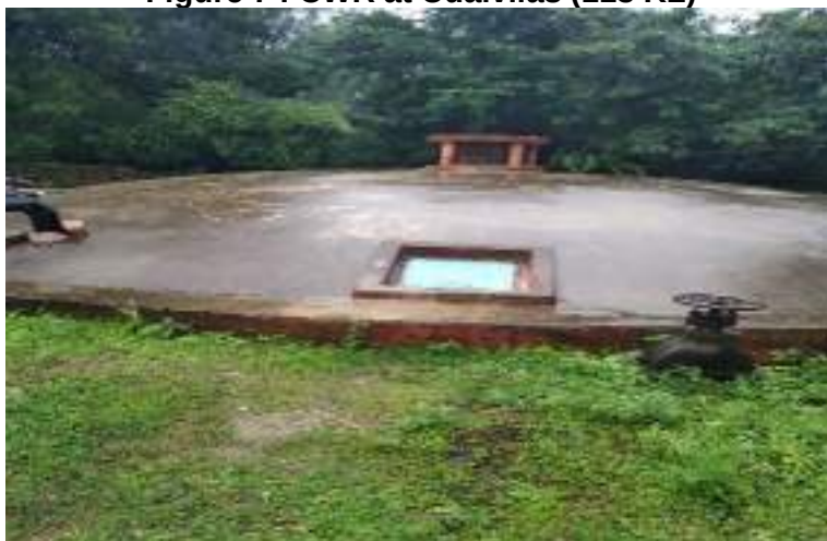
Figure 8 : CWR at Udaivilas (325 KL)
