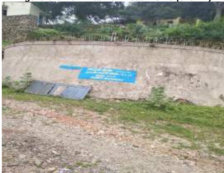
Figure 10 : Masonry CWR at AEN office (263 KL)
