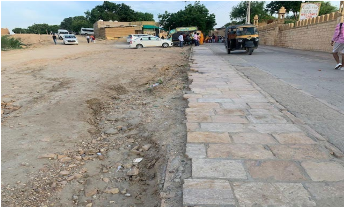
Location of the entrance plaza; existing road, sidewalk, erosion due to under managed stormwater
