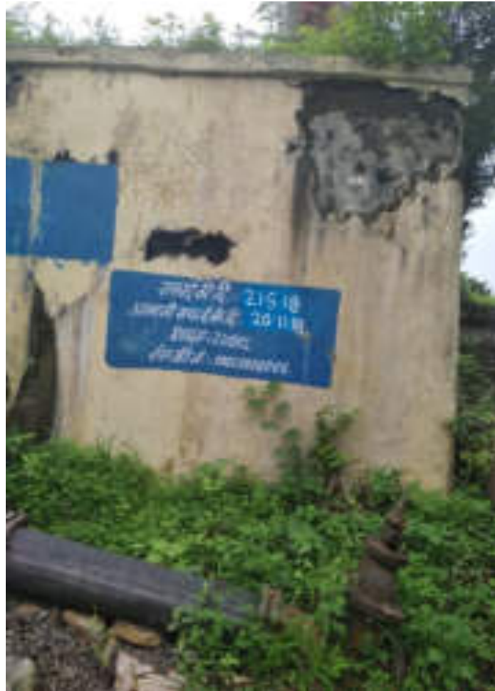
Figure 12 : Masonry GLSR for Ghati-I at hill near AEN office (200 KL)
