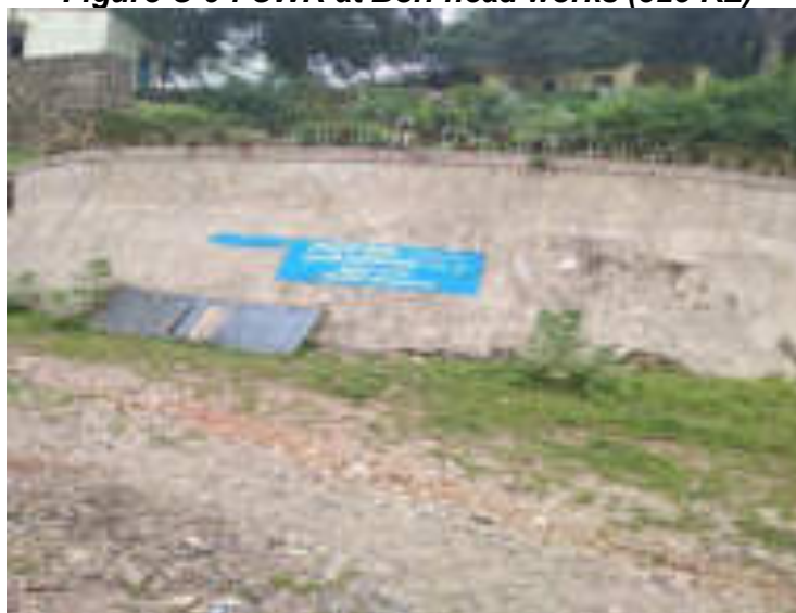
Figure 10 : Masonry CWR at AEN office (263 KL)
