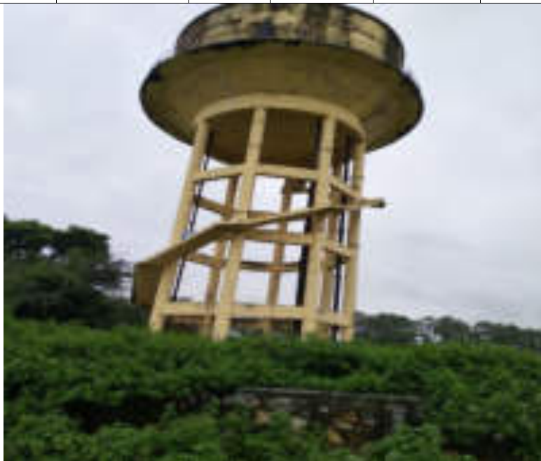
Figure 11 : Existing ESR at Navadera (325 KL)
