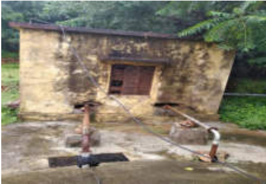
Figure 6 : CWR at Udaivilas (113 KL)
