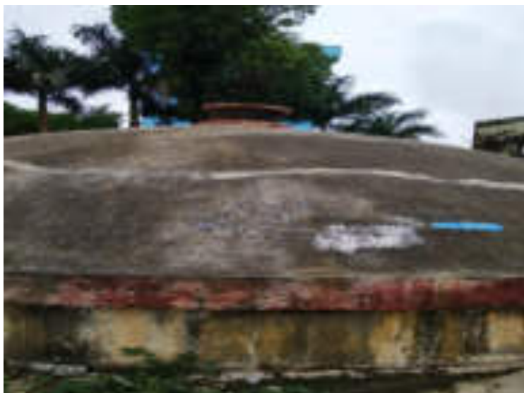
Figure C-9 : CWR at Bori head works (325 KL)
