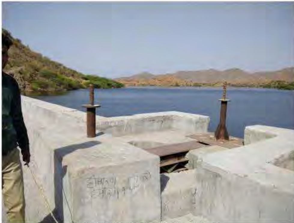
Photo 1 Valve to operate Gate of Bhaisa Singh Dam
