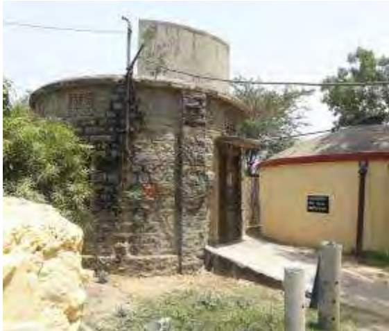
MARKET AREA PUMP HOUSE
