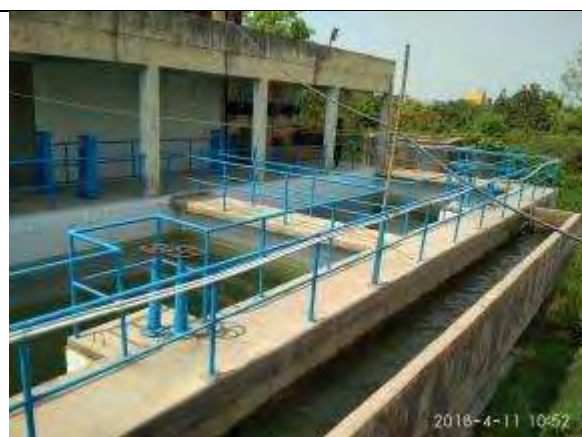
Existing WTP at AEN Campus
