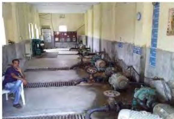
Main Pumping station near AEN PHED Office
