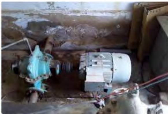
Pump House at Panchwa Road
