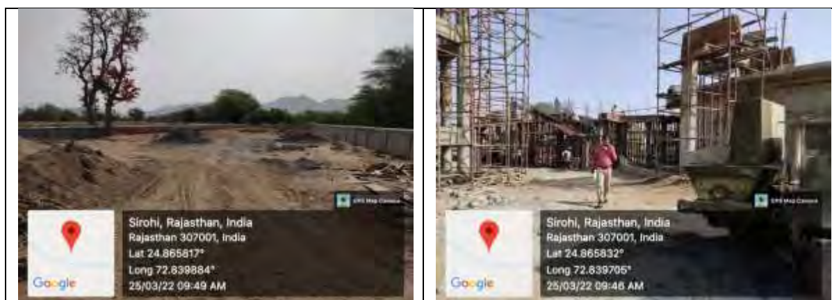
STP Site 1.7 MLD near Revdar Road, Sirohi
