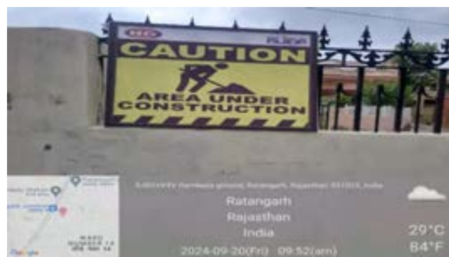
Good Practise: Display of Cautionary Board at site
