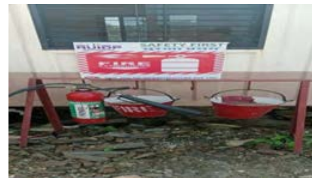
Good Practise: Display & Availability of Fire Extinguisher and Fire Bucket
