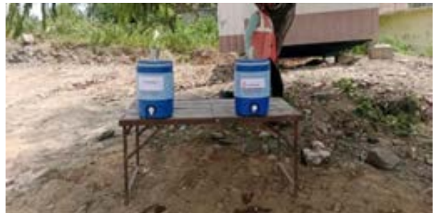
Good Practise: Drinking Water Facility At WTP Site
