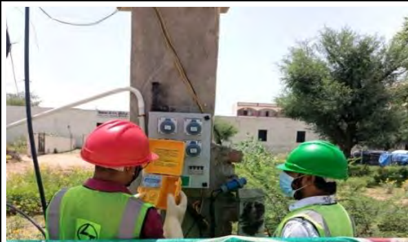
Good Practise Electrical
