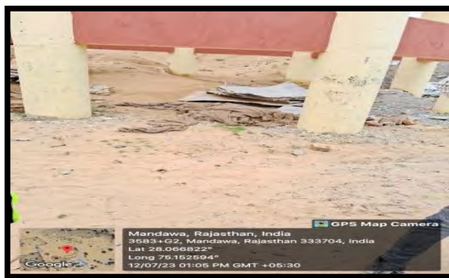
Loose sharp edges tin shed material was dumped without putting weight on it and unwanted debris material was dumped
