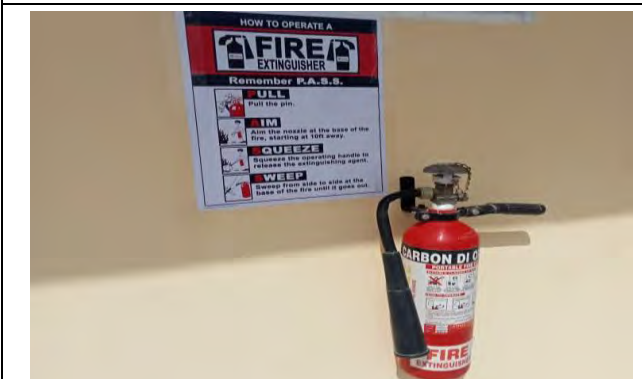
Good Practise Fire extinguisher at Site
