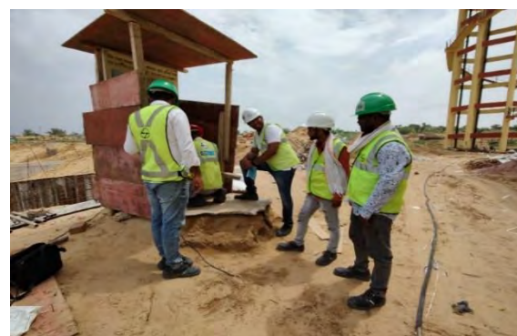
Good Practise Electrical (RCCB Testing)
