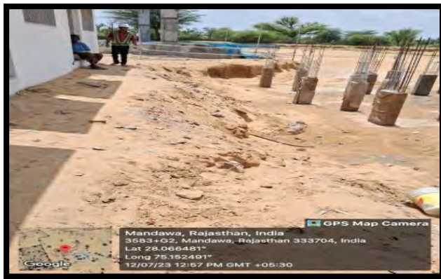
Uneven working area/platform was found in front of SBR area there may be chances that leads to slip/trip &amp; fall injury
