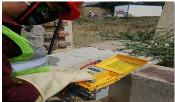
Good Practise Electrical
