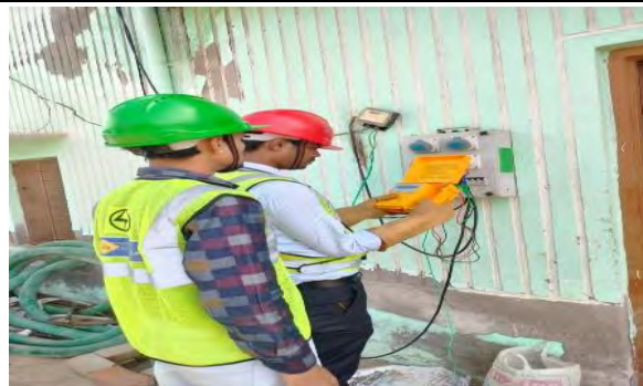
Good Practise Electrical
