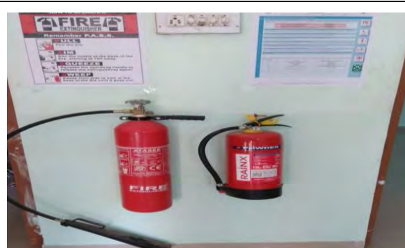
Good Practise Fire extinguisher at Site
