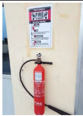
Good Practise Emergency No. Display & Fire extinguisher
