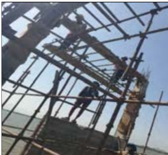
Worker found at WTP Intake 8.6 MLD angore without safety belt
