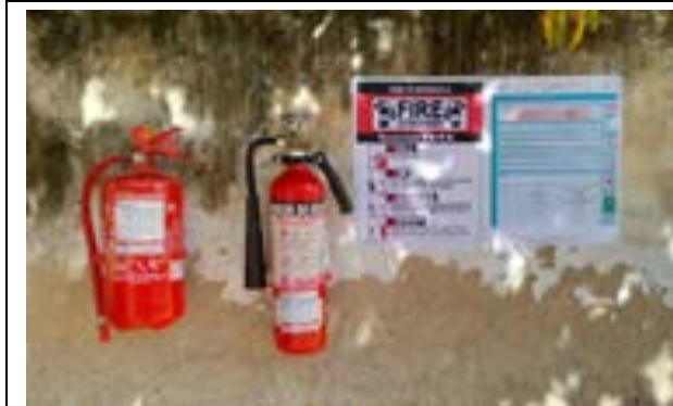
Good Practise - Fire extinguisher at Guest House
