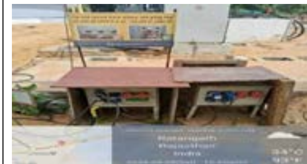
Good Practise Electrical Safety
