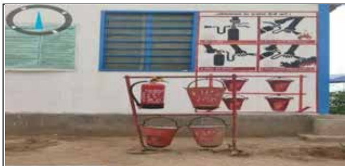
Good Practose - Fire extinguisher at Guest House
