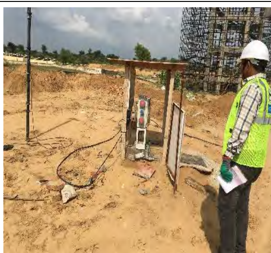
Good housekeeping at 2.3 MLD STP site, Sardar Shahar
