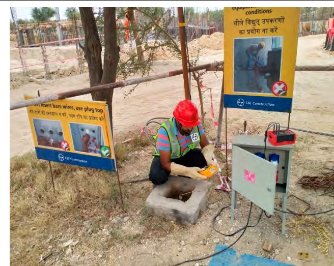
Good Practise Electrical
