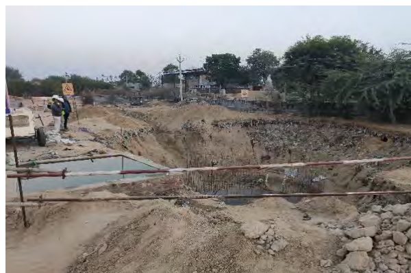
No helpline number is display on information board at SPS Site Behind Dholi Sati Temple
