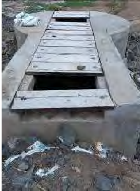
Manhole with Pumping (MwP) 0.10 MLD within the earthen right of way (RoW) of existing road (Manpur road) belongs to NP-Pratapgarh town.
