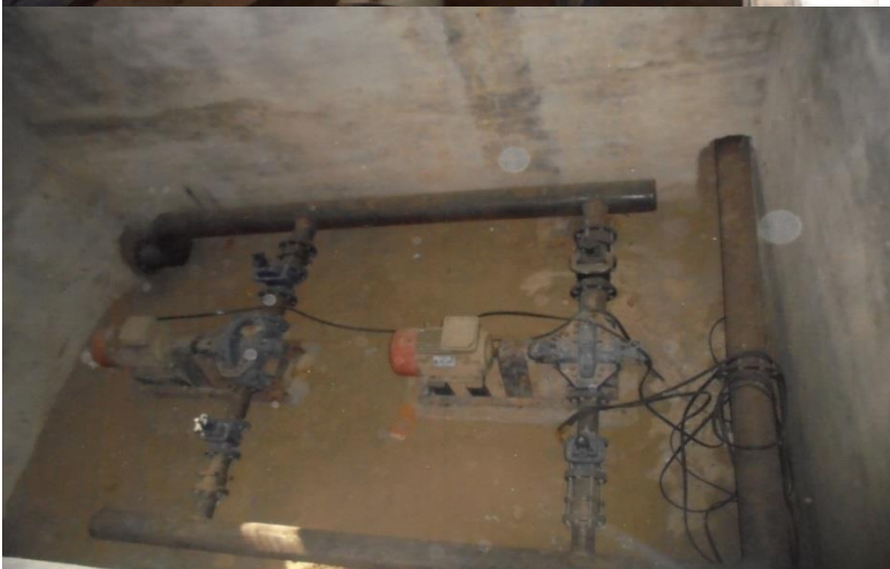
Clear Water pumps at Zone -6 pumping station
