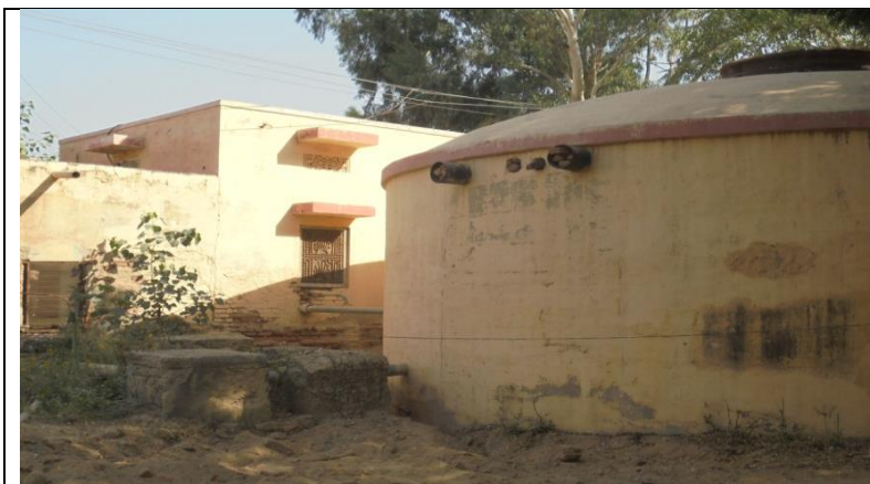
Spots of leakage in GLSR wall
