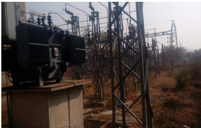
AIS Switch yard at OLD CWPH
