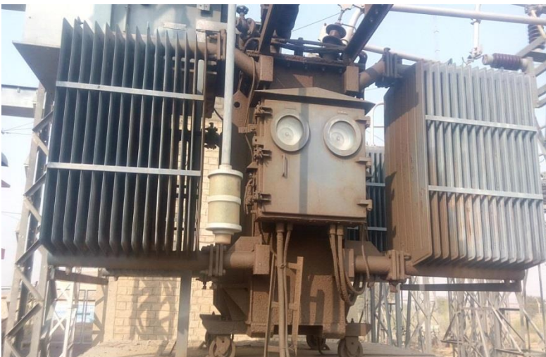
Transformer at SADASAR
