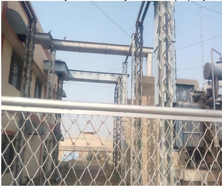
AIS switchyard at PALOO
