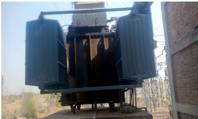
Transformer at Pallu
