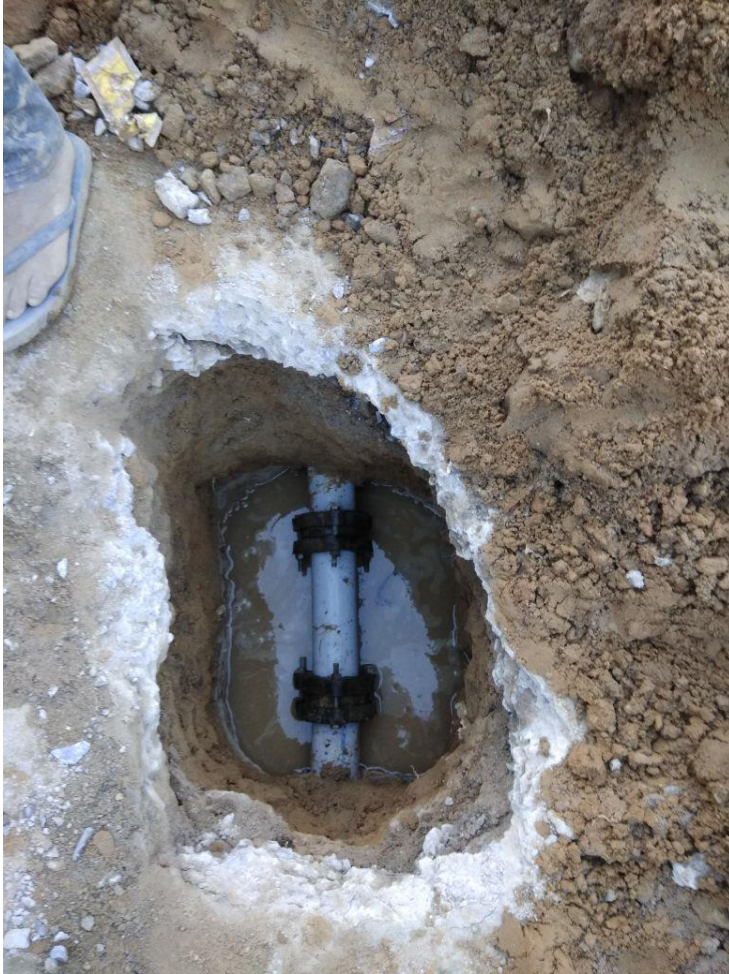
Leakage at Existing Distribution Network uPVC line, at Ward No- 06
