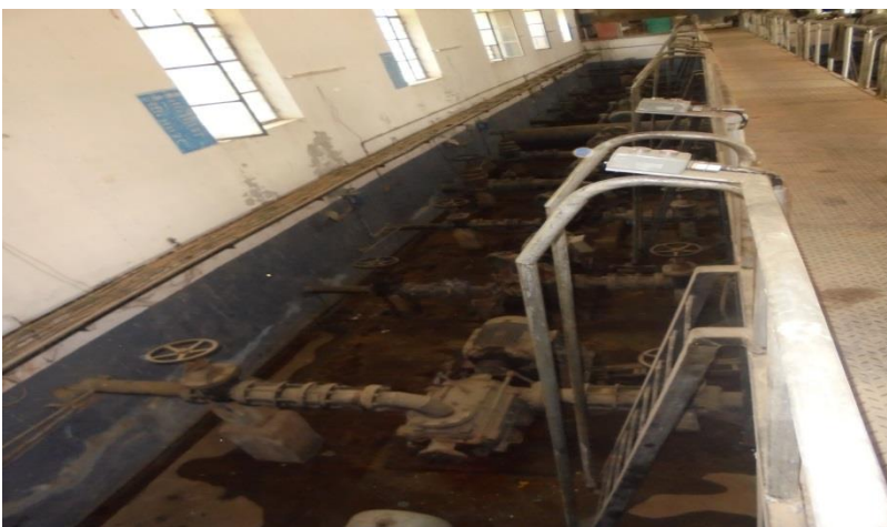
Clear water pumps at CWPS
