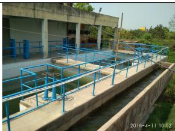
Existing WTP at AEN Campus
