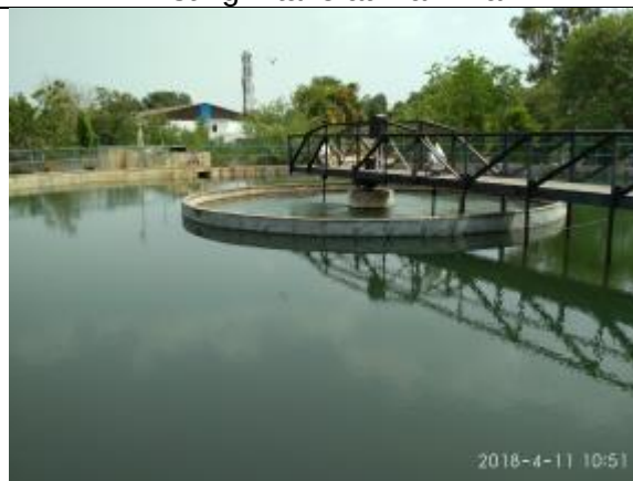
Clariflocculator at Existing WTP at AEN Campus
