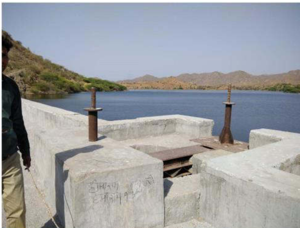
Photo 1 Valve to operate Gate of Bhaisa Singh Dam
