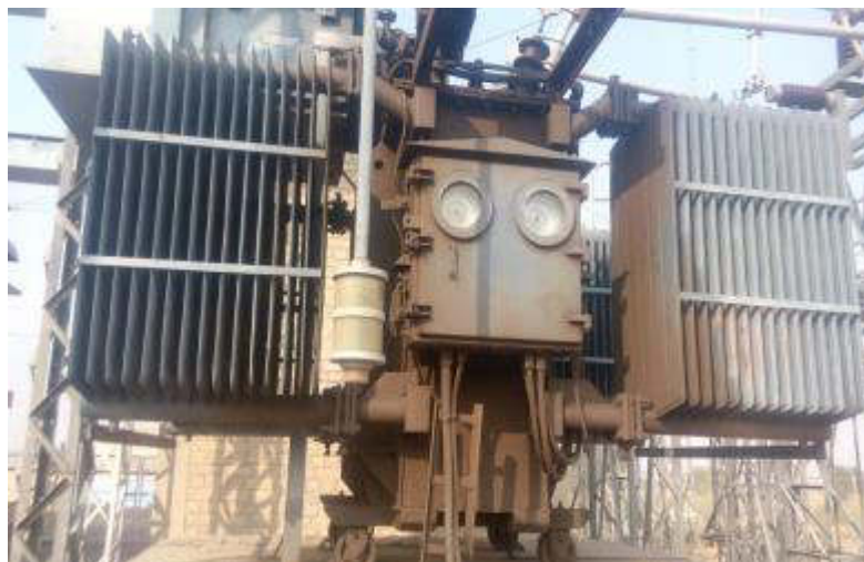
Transformer at SADASAR
