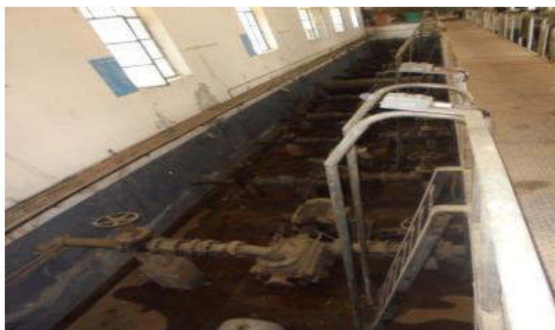
Clear water pumps at CWPS
