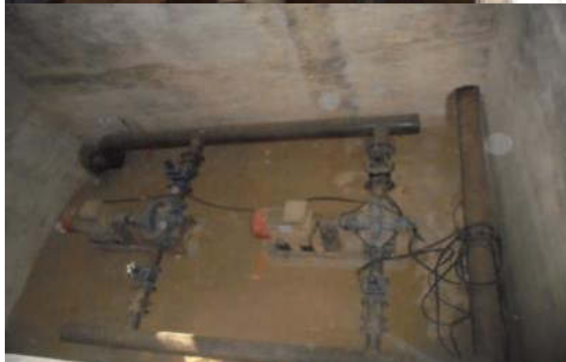
Clear Water pumps at Zone -6 pumping station
