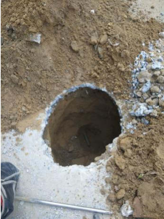
Distribution Pipe Line located at an depth of more than 10ft at Ward No-15.
