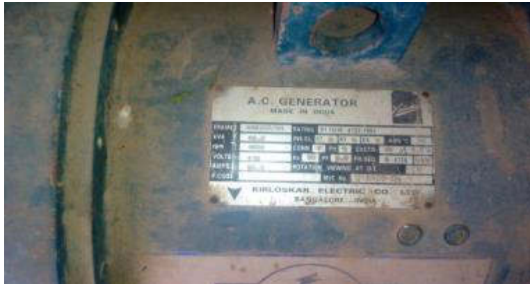
DG SET at OLD CWPB
