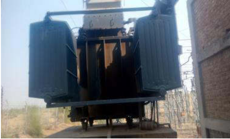
Transformer at Pallu
