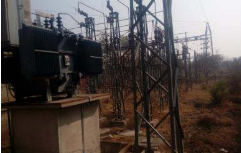
AIS Switch yard at OLD CWPH
