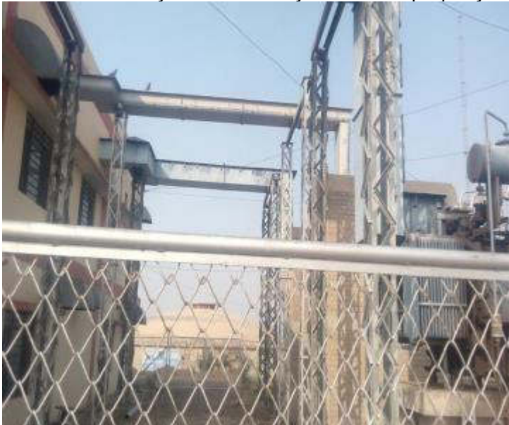
AIS switchyard at PALOO
