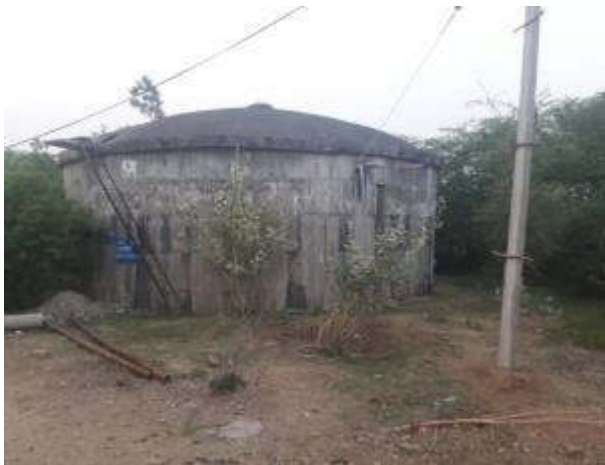
RAMPURA PUMP HOUSE (RAMPURA PALDI) HOUSE(SADULPURA)
