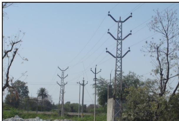
Photo 5: Electrical utilities coming on access road needs to be shifted
