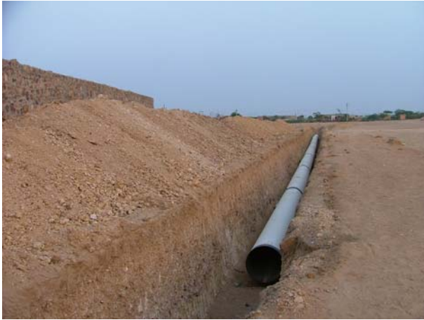
Water Pipe line for Barmer Water Supply
