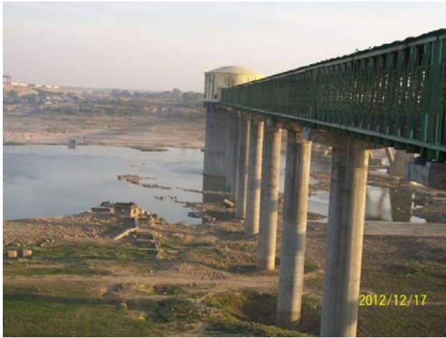
Intake well Structure of Public Health & Engineering Department at Dholpur
