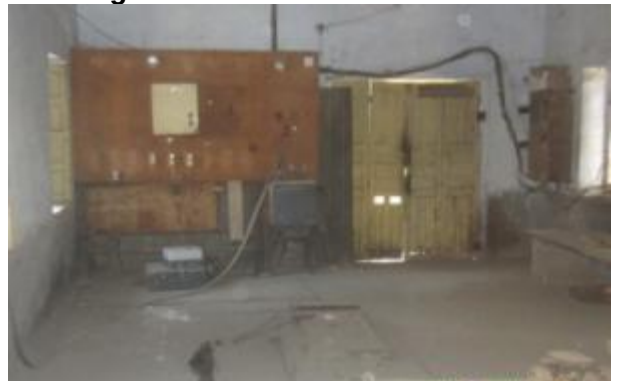
Conditions of Pump
