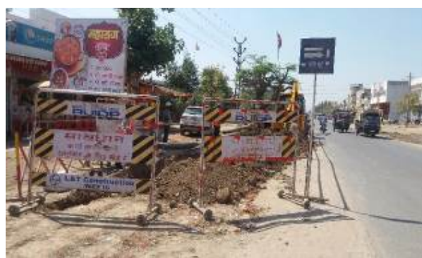
Water supply pipeline with proper barricading and access availability
