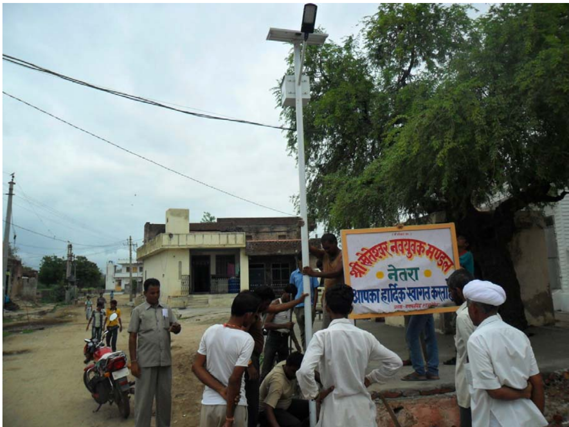
Figure 3.1: Solar Light Installed in Netra as Part of EPA
